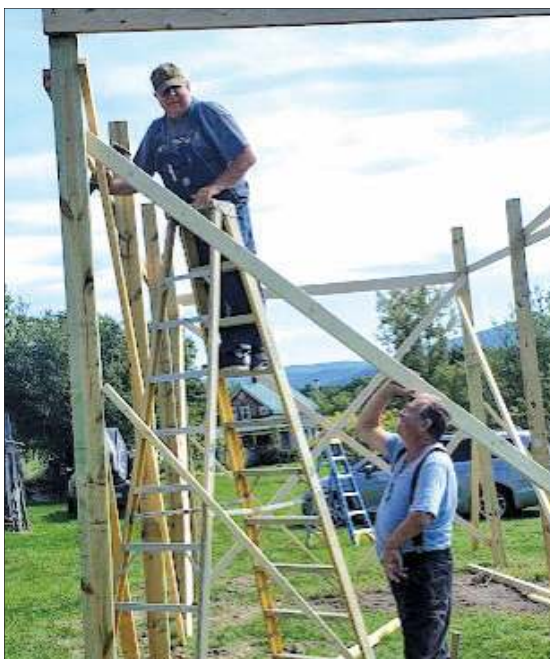
TODD NIELSEN AND his father, Stanley (on ladder), working on a pole barn at Todd's house on Corona Street in Brandon.
