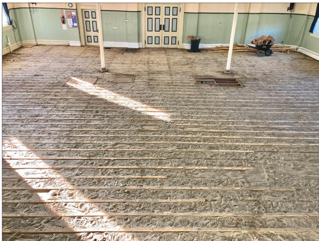
WHEN THE EXISTING floorboards were pulled up, the spaces between the joists were found to be filled with sand, a decidedly low-tech method to muffle sound when that floor was installed. All the sand had to be shoveled out, filling an entire dump truck, before the new subfloor could be installed.
