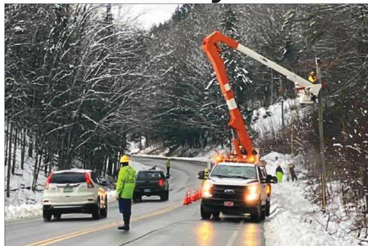
HARDWICK ELECTRIC DEPARTMENT staff repair damaged power lines along Route 14 in Hardwick on Monday, Nov. 27.
