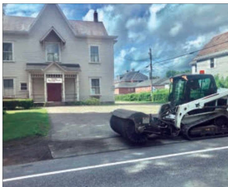
THE SIDEWALK IN front of the Pittsford Historical Society is prepared for temporary paving in anticipation of the Segment 2 overhaul of Route 7 in Pittsford Village. Photo by Steven Jupiter
